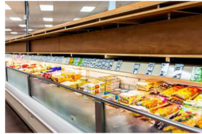
Open air refrigeration in a grocery store
